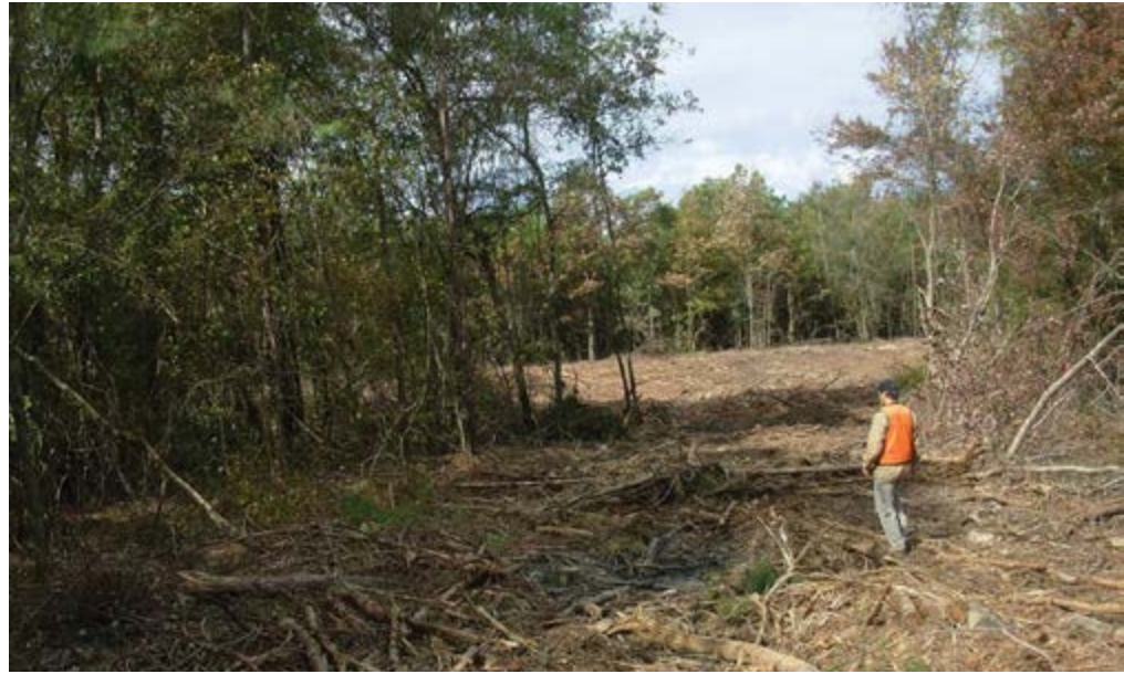
This stabilized, temporary creek crossing is covered with slash to protect the stream until natural vegetation can regenerate.
